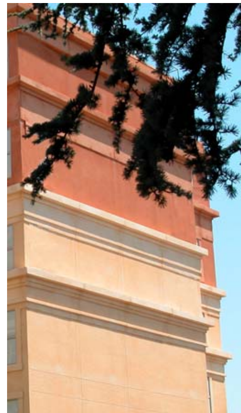
Example of poorly articulated and blank facade
