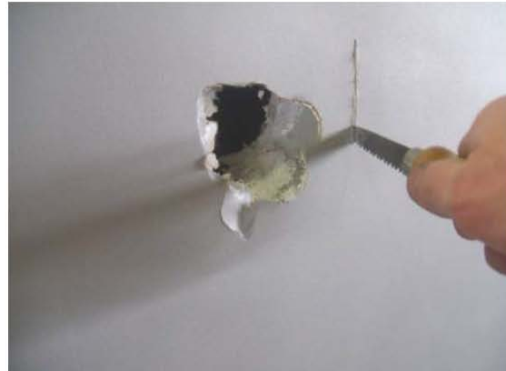
Figure 2: Square Off Damaged Area
