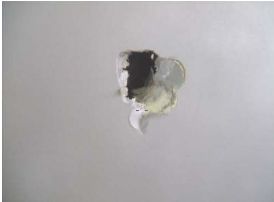
Figure 1: Damaged Gypsum Panel
