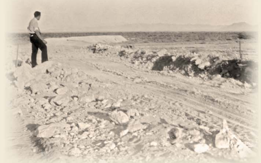
A worker looks toward Sunset Park and Railroad Pass from the junction of the Boulder Branch Railroad and the Union Pacific main line. - Boulder City Museum and Historical Association, Elton and Madelaine Garrett Collection
